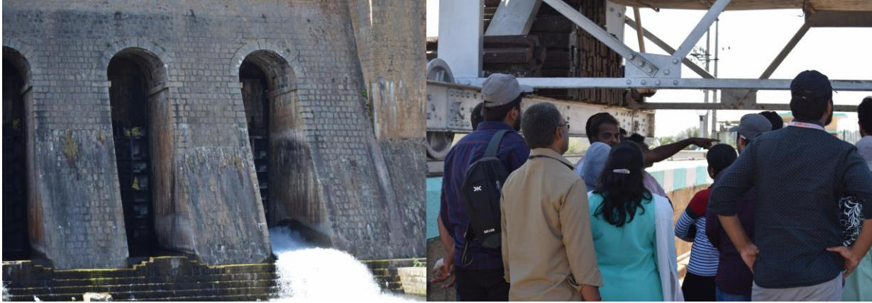
Sluice gates and Emergency sluice gates slider
